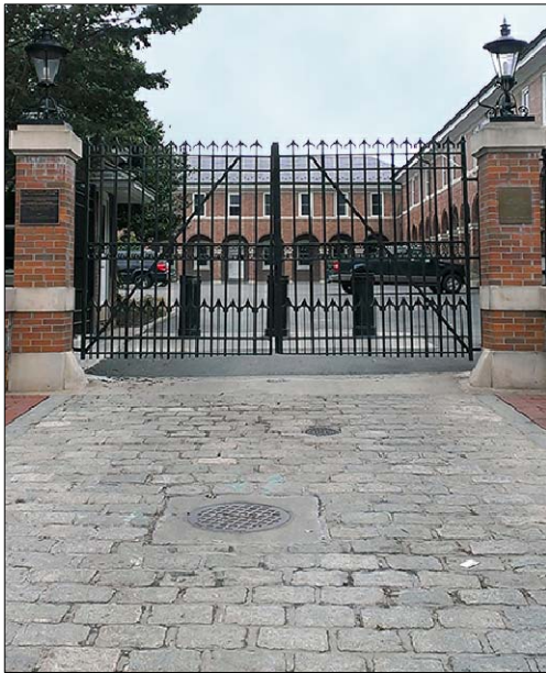
MAIN GATE DRIVEWAY ISSUE: UNEVEN PAVEMENT Image: existing entrance, granite setts, March 2014
